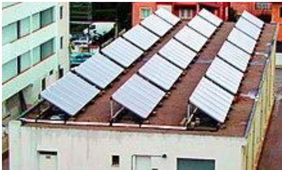
Solar collectors for domestic hot water preparation at a hotel in Mallorca.
